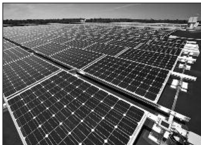
PHOTO: THE UNIVERSITY OF MARYLAND OFFICE OF SUSTAINABILITY COMMUNICATIONS A display of 2,600 solar panels are displayed atop the Severn building at the University of Maryland. Photo courtesy of the University of Maryland Office of Sustainability Communications
