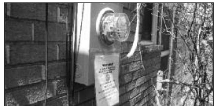
Jonathan Libber's analog electricity meter sports a no-replace notice for BGE employees.
