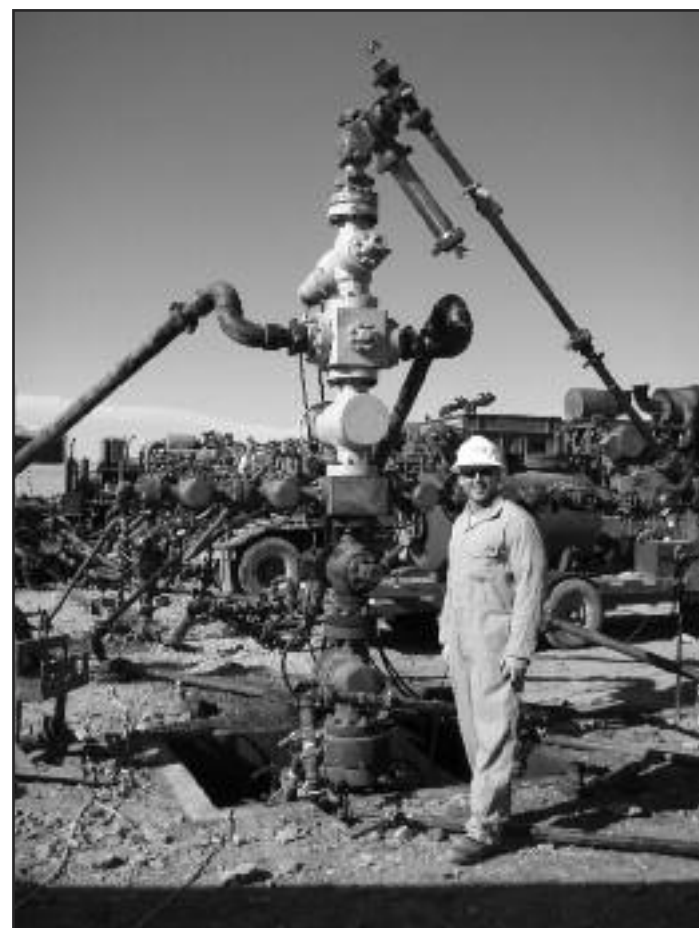
Well Head where fluids are injected into the ground.
